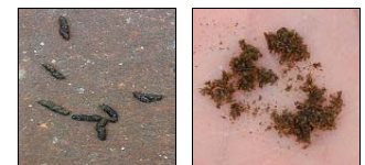
Bat droppings crumble to dust
